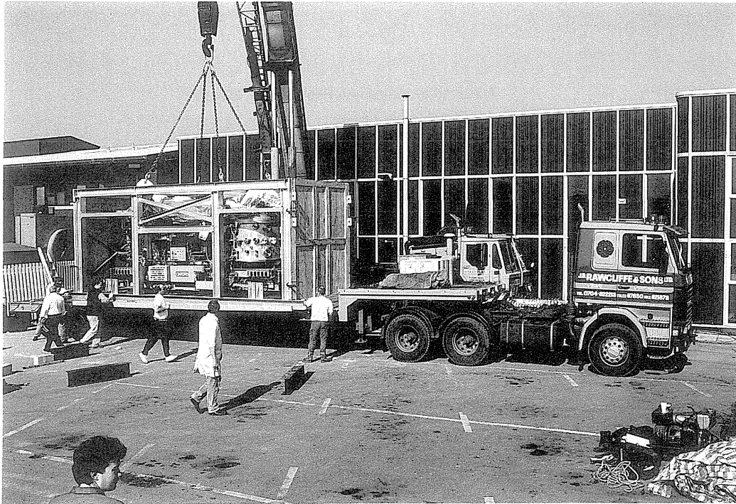
Fig.1 HELIOS 1 on lorry leaving Oxford for East Fishikill, transported as one assembled unit.
